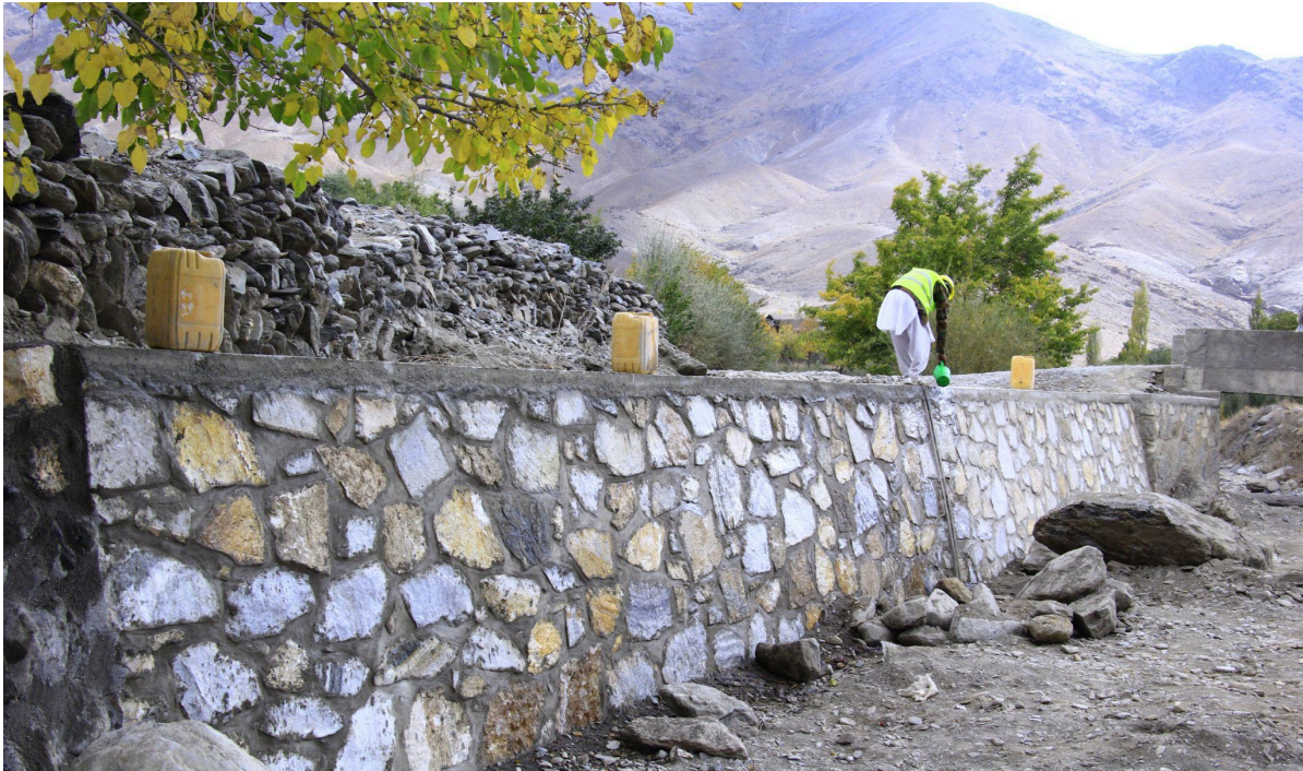
A new protection wall in Afghanistan's Wardak province will help protect the local community from flooding. ©UNOPS/Rafiullah Hemat
