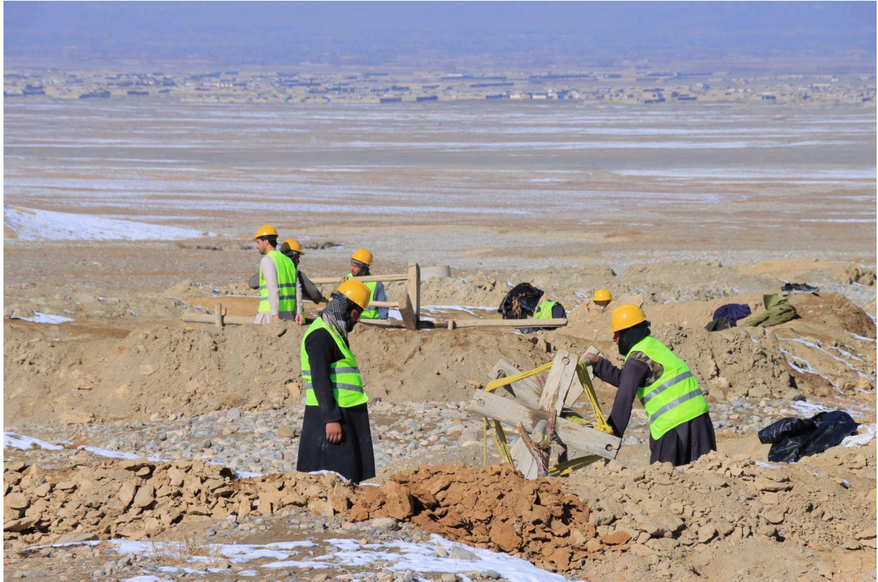
Afghans working to rehabilitate vital underground water reservoirs in the country's Logar province. ©UNOPS/Rafiullah Hemat
